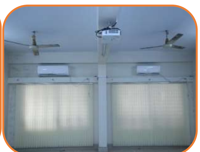
CEDP Funded Air-Conditioning Equipment in the Laboratory
