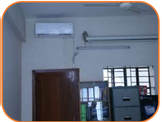
CEDP Funded Air-Conditioning Equipment in the Laboratory
