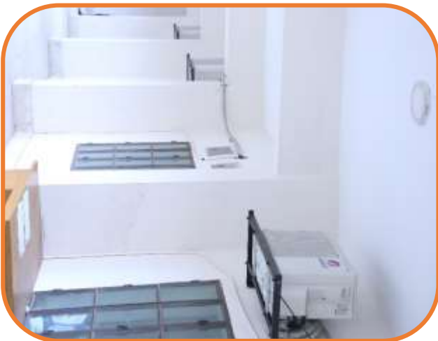
CEDP Funded Air-Conditioning Equipment in the Laboratory
