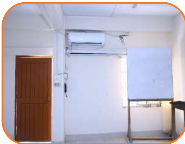
CEDP Funded Air-Conditioning Equipment in the Laboratory
