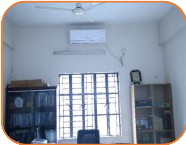
CEDP Funded Air-Conditioning Equipment in the Laboratory
