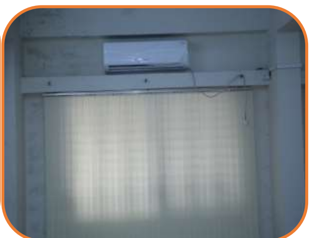
CEDP Funded Air-Conditioning Equipment in the Laboratory
